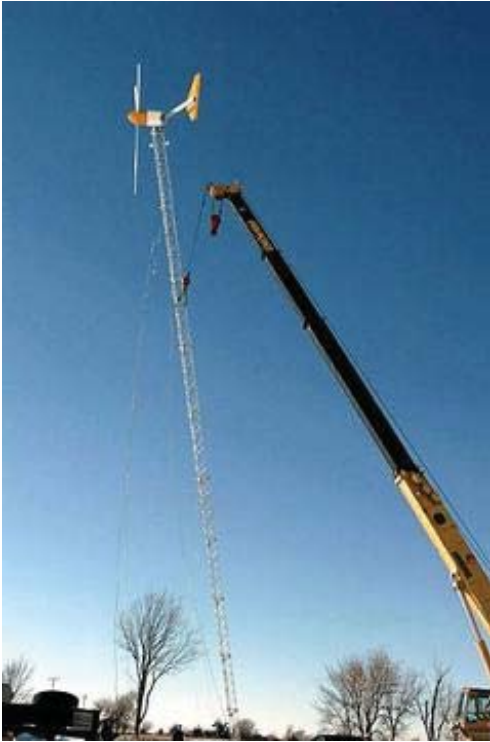
The turbine was attached to a 100-foot guyed lattice tower and hoisted into place adjacent to an existing GCW.
