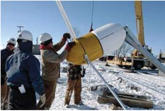
The turbine manufacturer provided personnel to assist in turbine installation and electrical equipment setup. GCW retrofit included installation of a new circuit box enabling the system to operate in grid inter-tie mode.
