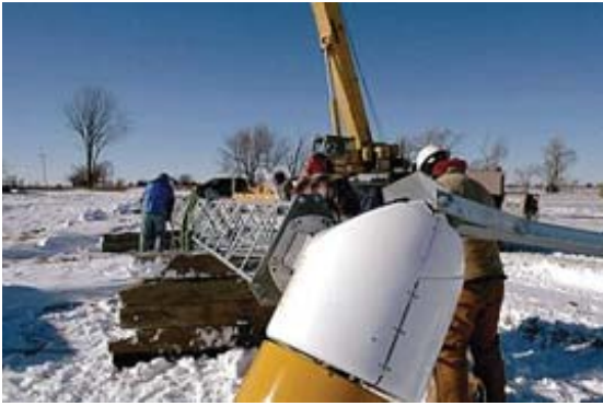
The 10-kW Bergey Excel S wind turbine system arrived at the site in December 2003.
