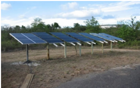
Selection of fixed-position modular panels allows easy expansion to accommodate additional enhancements to the fluid gathering system.
