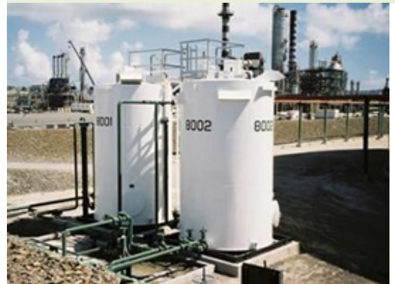
Recovered subsurface fluid accumulates in aboveground tanks at the adjacent HOVENSA oil refinery, where separated oil is used as refinery feedstock.
