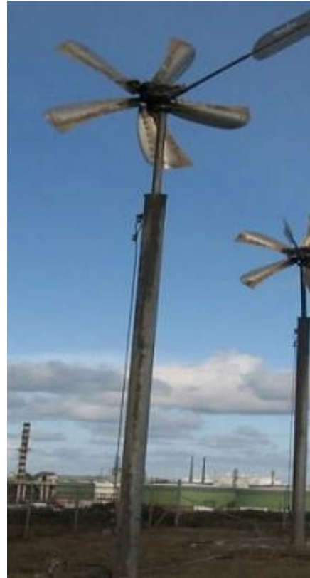
Each wind turbine compressor is powered by a windmill with 4.3-foot blades that begin rotating at a wind speed of 4 mph. The air compressor is located directly behind the windmill on a hinged tower.
