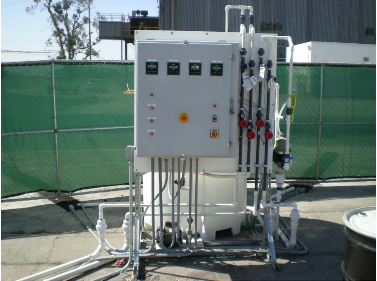
Picture 19. Surge tank and control panel front.
