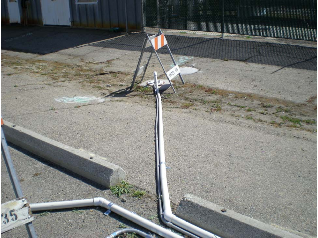
Picture 12. Piping to AIW-2.
