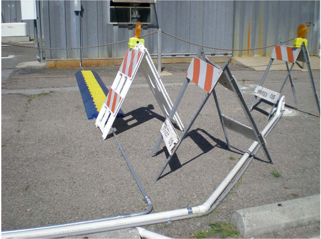
Picture 11. Piping to AIW-1.
