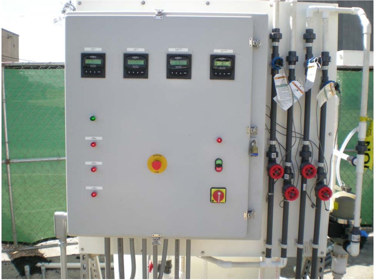
Picture 3. Injection system control panel.
