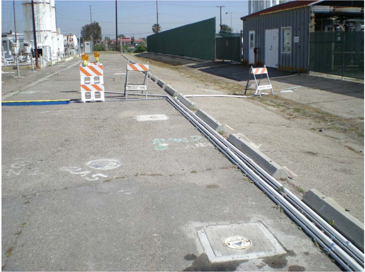
Picture 14. Piping between injection and extraction wells.
