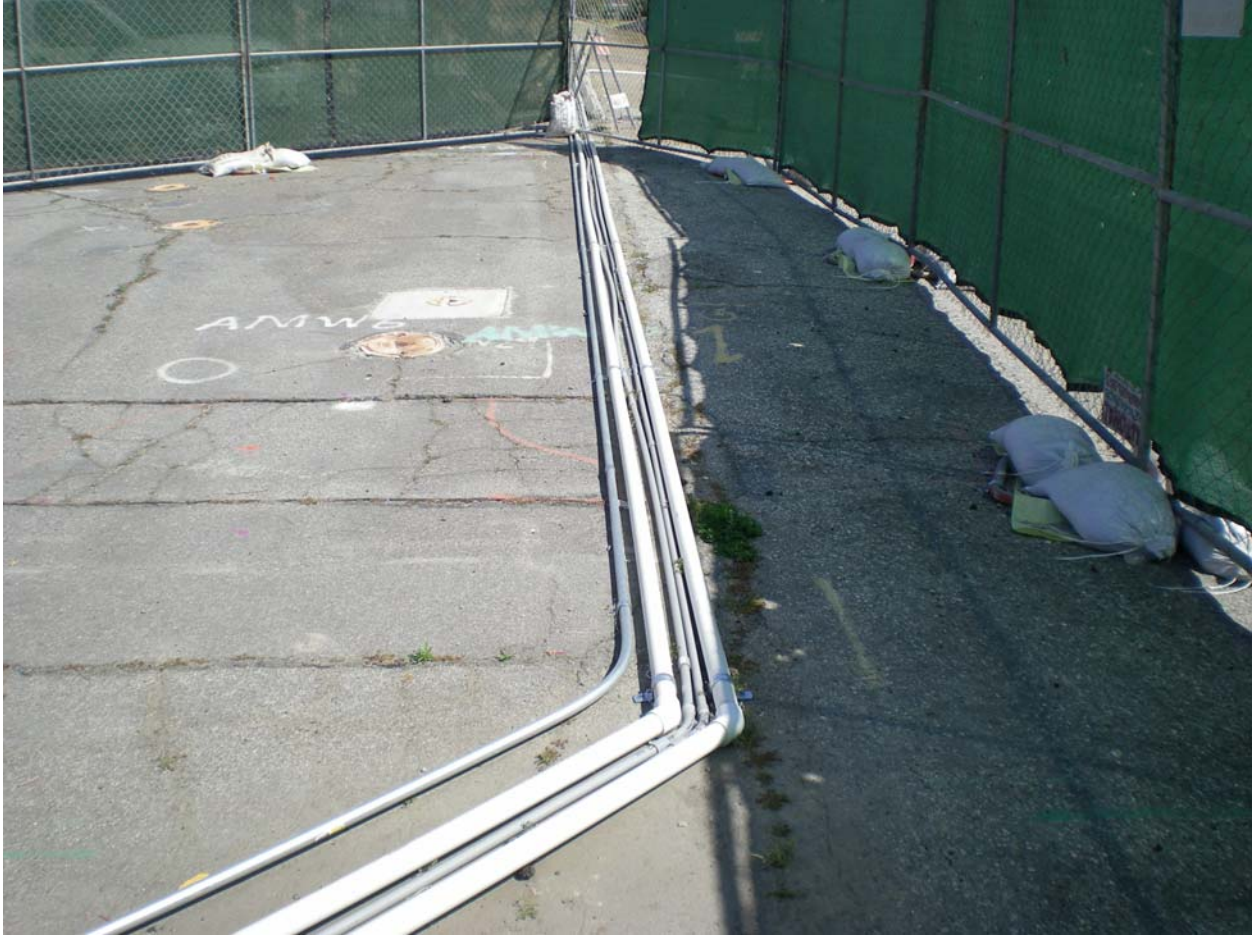
Picture 13. Piping between injection and extraction wells.
