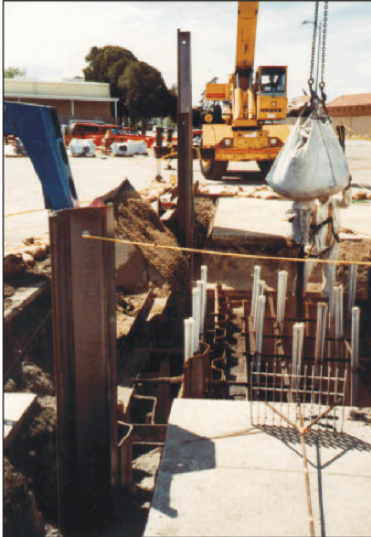
Figure 7-2. Placement of Reactive Iron Media (Suspended Bag) and Pea Gravel (Front-End Loader) into Divided Sections of Trench for a PRB (Courtesy of PRC, 1996)
