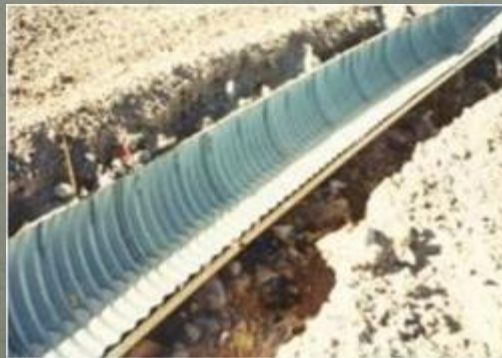
Poor Surface Water Controls
