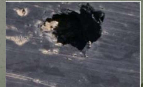
HDPE Liners – Easily Damaged
