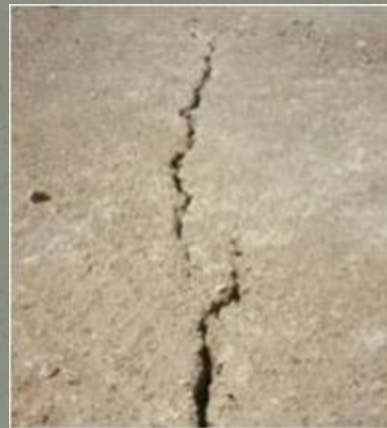
Tension Cracks Perpendicular to Surface Water Flow
