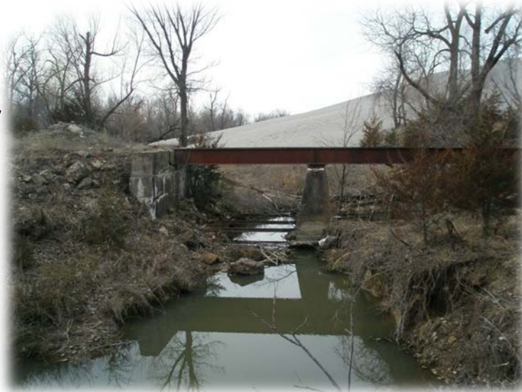
Example of Bank Erosion
