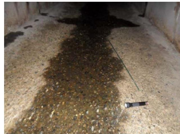
Erosion of Concrete Approximately 1" Deep
