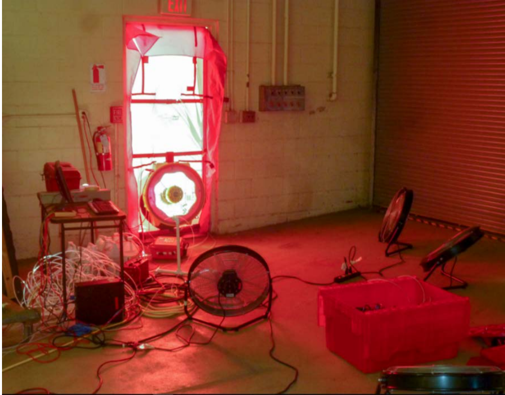
Figure 4. The blower door installation and the air mixing near blower intake with floor fans.
