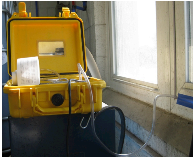
Figure 3: Example Pressure Transducer Installation
