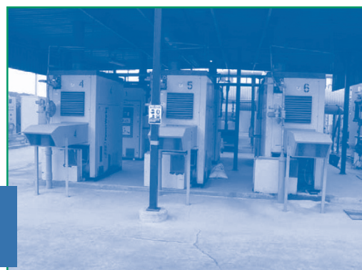
Figure 3. OII's microturbines were installed in a covered area immediately adjacent to the LFGTP.
