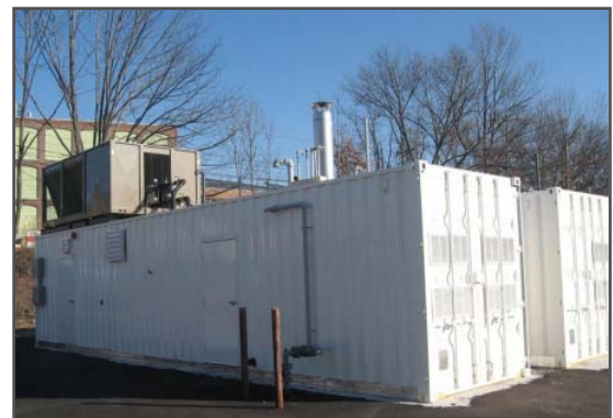
Figure 5. Storage units containing the synthetic media system used at the Waltham site.
