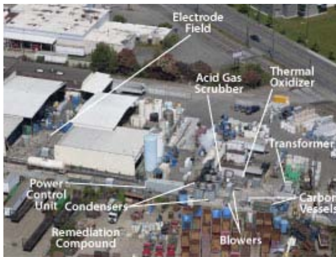
Figure 1. Locations of ERH electrode field and supporting remedial equipment at the Fox Avenue site.
