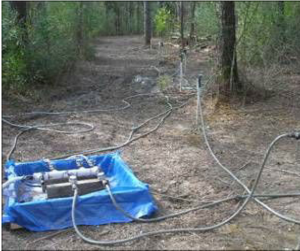
Figure 1. Delivery of substrate from a single 500-gallon tank into four injection points via a positive displacement pump.
