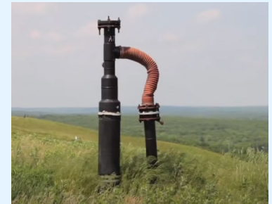
The 154-acre Central Landfill site is located within the Central Landfill, an active municipal solid waste disposal facility in Johnston, Rhode Island. This NPL site encompasses an area formerly used to dispose of hazardous industrial wastes. Site cleanup has involved constructing a multi-layer cap and hydraulically containing and treating underlying groundwater. A gas-to-energy plant has operated at the landfill since 2013, with a current capacity of about 33 MW. The capped area, a portion of which is now buried by newer waste, has contributed up to 12 percent of the total LFG collected at the landfill.
