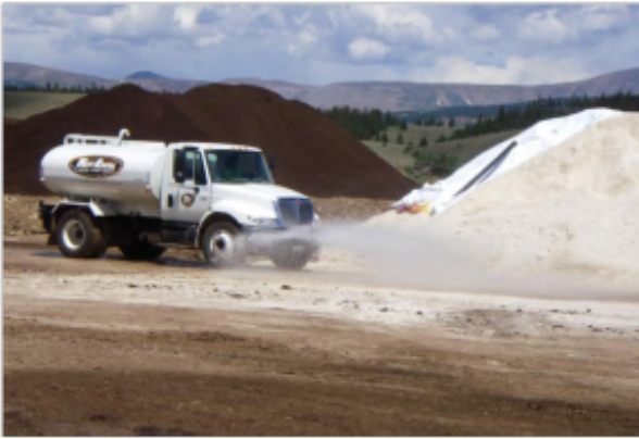
Approximately 7,000 tons of sugar beet lime was mixed into the soil prior to compost application. A precision hydraulic mixer was used to assure coverage along uneven boundaries and around large (up to 12-inch) rocks.
