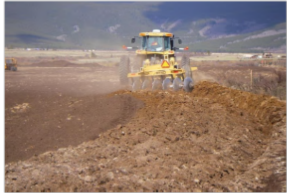
Approximately 14,000 tons (23,000 cubic yards) of compost were mixed directly into the upper soil.
