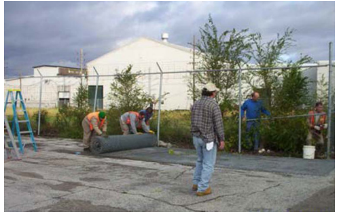
Fencing Reuse: Volunteers dismantled and removed 8-foot chain link fencing no longer needed at the main plant area and re-installed it in certain sections of the regional Nickel Plate recreational trail.
