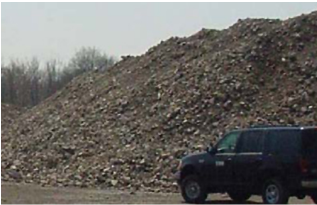
Concrete Salvaging: Demolition concrete was crushed onsite and stockpiled for use as fill at the main plant area after its excavation was complete.
