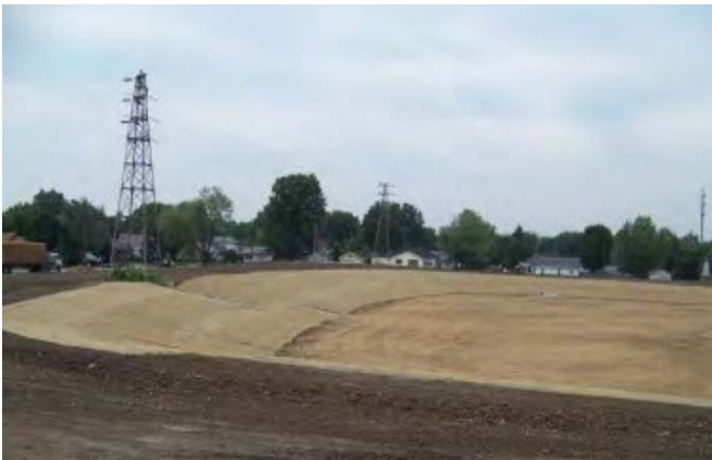
Stormwater Management Infrastructure: The onsite stormwater retention pond created in the former quarry area collects clean stormwater accumulating on the site as well as stormwater diverted from adjacent neighborhoods. (photo source: IDEM)
