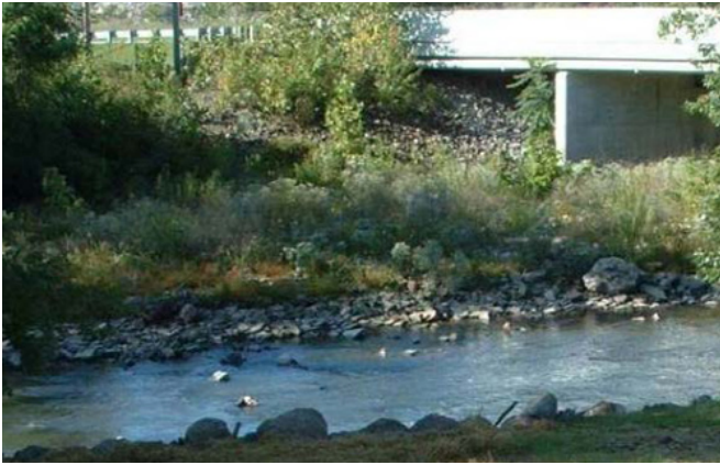
Creek Bank Armoring: Large granite field stones were extracted from imported clean fill and used to stabilize onsite banks of Kokomo Creek and Wildcat Creek, which runs below a local transportation corridor (Dixon Road).
