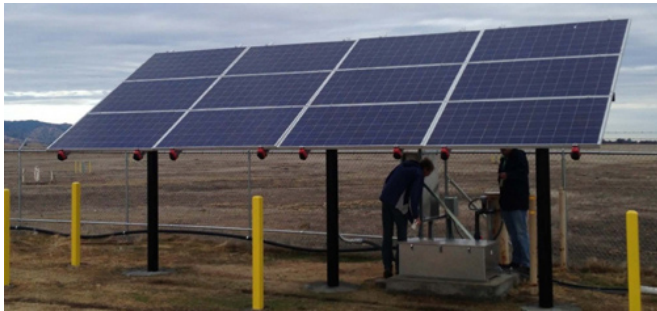
Site LF007C PV System: The ground-mounted PV array supporting P&T operations at Site LF007C consists of 12 panels equipped with a storage battery.
