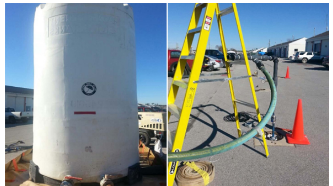
Site 78 Injection: ERD at Site 78 involved gravity-feed injection of EHC® Liquid ISCR reagent, which includes a controlled-release organic carbon substrate and an organo-ferrous compound (both of food grade). The same substrate was injected via gravity feed at Site 89.
