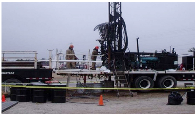
Rotasonic Drilling: When compared to a conventional rotary or auger drilling process, rotasonic drilling typically requires less power to operate and generates less soil friction immediately adjacent to a drill string.
