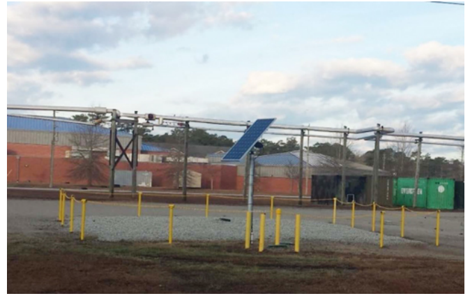
Biogeochemical Reactor: At Site 93, a pump powered by a co-located photovoltaic array recirculates contaminated groundwater through a subsurface reactive cell.
