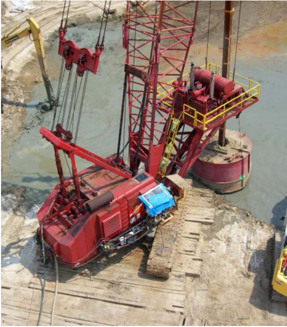
In Situ Soil Mixing: A crane-mounted drill rig was deployed for soil mixing at Site 89. A 10-foot-diameter mixing auger was used to drill, inject ZVI and bentonite clay slurry at the mixing head, and mix the materials to produce a homogeneous soil column. The mixture was applied at specific ratios in three designated areas to a depth of 25 feet.
