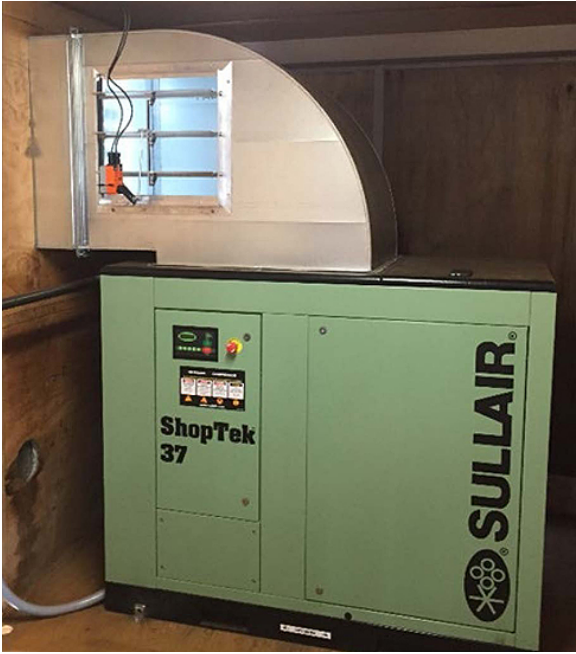
Equipment Reuse: Air sparging equipment no longer needed at either of two sites was reclaimed for future use at other Camp Lejeune sites. Shutdown of air sparging operations upon reaching risk-based cleanup goals saved approximately 800,000 kilowatt hours of electricity per year at each site.
