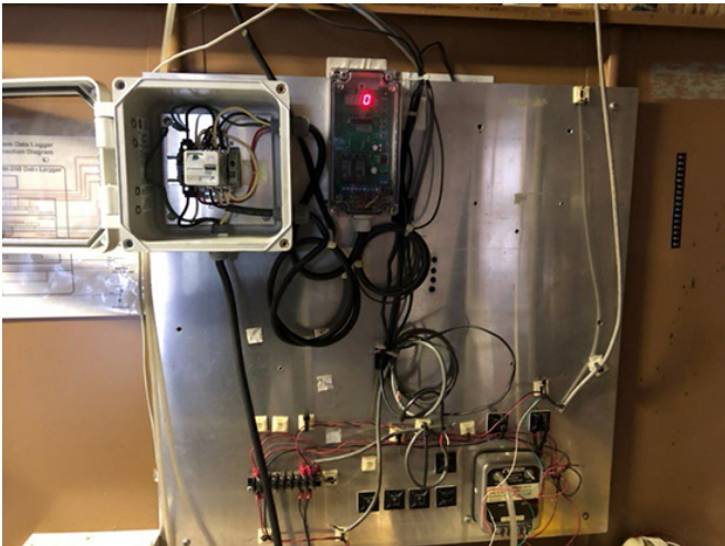
Windmill Controls: The automatic brake system includes a wind speed gauge and power/fuse box inside the building adjacent to the windmill.
