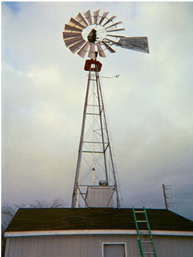
Co-Located Equipment: Equipment for managing extraction of the landfill gas and operating the onsite windmill is housed inside a 150 square-foot building adjacent to the windmill.
