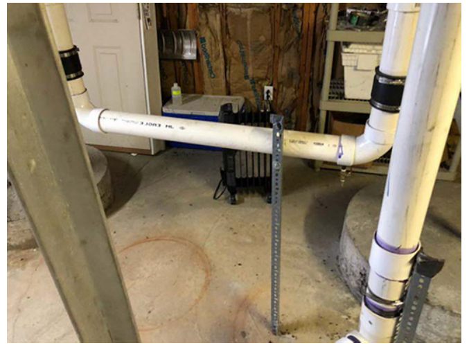
Transfer of Extracted Air: The extracted air flows through piping in the small building before it is discharged near the top of the windmill. This configuration provided weather-resilient housing for GAC canisters that were required to treat soil vapor during the initial nine years of SVE operations. It also provides space for canister reinstallation if needed in the future.
