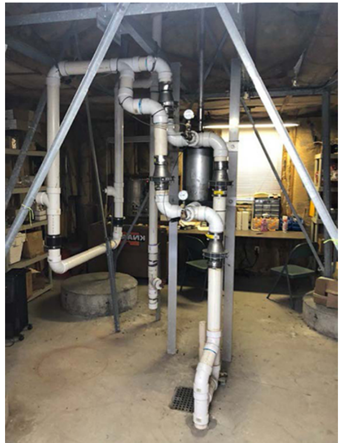
Air Cylinder System: Check valves installed on each side of the SVE air cylinder enable vacuum generation during both up and down strokes of the windmill.
