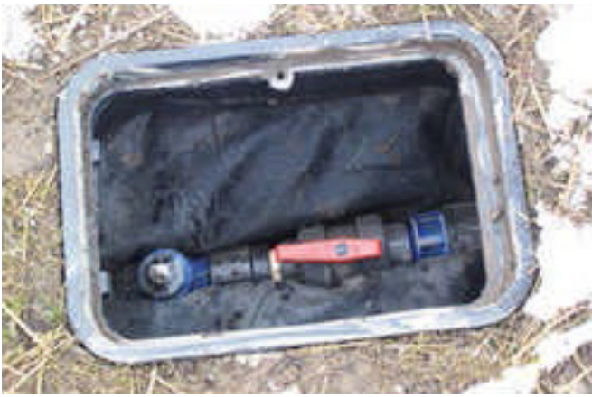
Vacuum Controls: A subsurface valve box at each gas vent is used to control vacuum throughout the landfill and as a sampling point.
