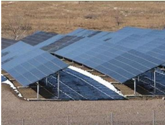
More than 27,000 panels comprising flatplate, thin-film solar technology were installed on the cap surface and other areas over several months in 2007.
