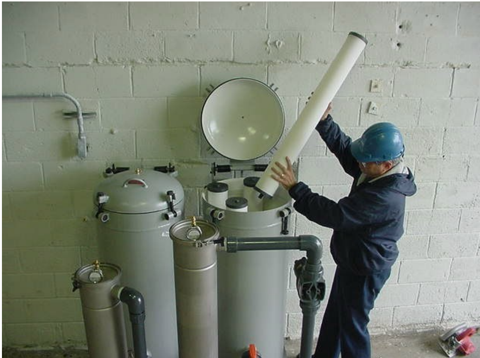
Figure 2-1D. 150-gpm Isolux ™ -302M Media Arsenic Adsorption System by MEI (Nine Replaceable Media Cartridges in Each Carbon Steel Vessel)
