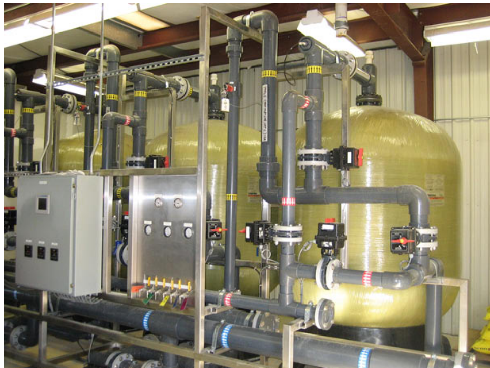
Figure 2-1F. 450-gpm E33 Media Arsenic Adsorption System by Severn Trent Services (Three FRP Vessels in Parallel)
