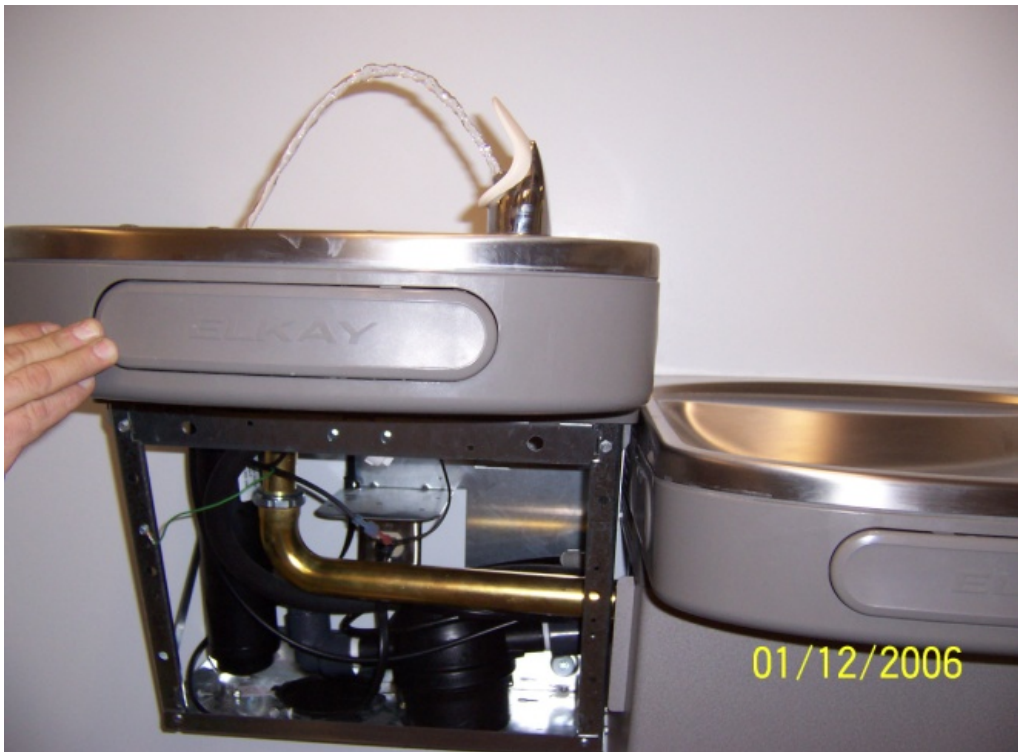
Figure 4-4. POU AM Units Installed Under a Sink (top) and Inside a Drinking Water Fountain (bottom)
