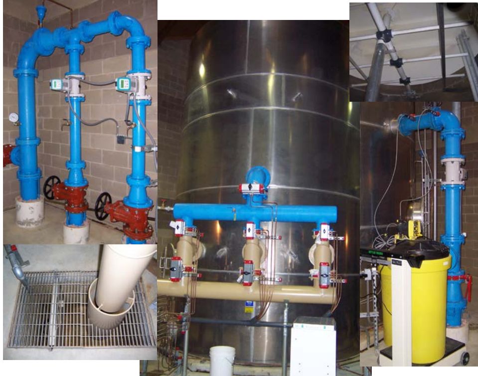
Figure 3-1E. 340-gpm AERALATER® Filtration System by Siemens (Clockwise from Left: Inlet Piping from Wells; Air Diffuser Grid within Detention Tank; Prechlorination Equipment; AERALATER® Unit with Detention Tank and Gravity Cell Influent; and Discharge Piping)
