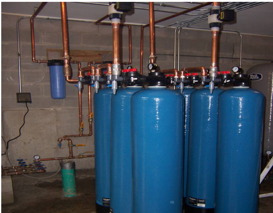
Figure 2-1B. 14-gpm As/I Complex 2000 Media System by ATS (Two Trains of Three Polyglass Vessels in Series)
