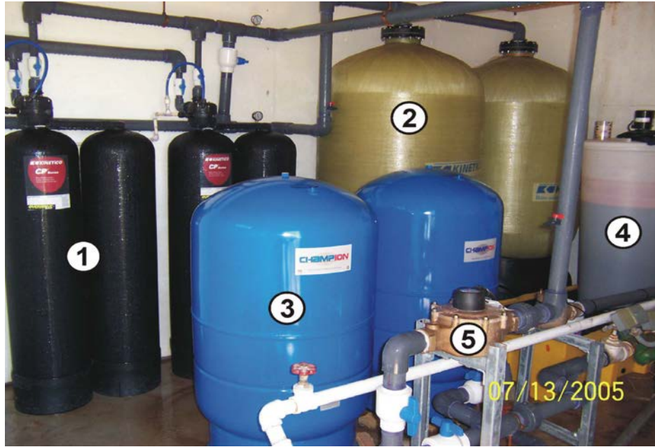
Figure 3-1A. 20-gpm Macrolite® Pressure Filtration System by Kinetico (1. Duplex Units, 2. Contact Tanks, 3. Pressure Filters, 4. Chemical Day Tank, and 5. Totalizer on Raw Water Line)
