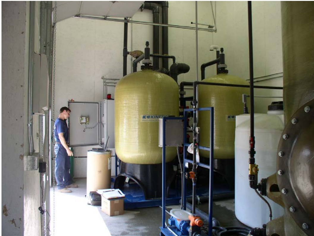
Figure 4-1. Photograph of IX-248-As/N System at Fruitland, ID
