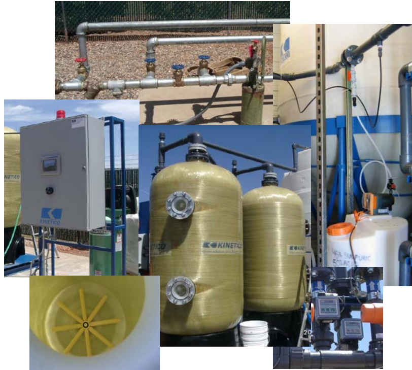
Figure 2-5. AM Treatment System Components at VV by Kinetico (Clockwise from Top: POE Well No. 2 and Bypass Piping; Acid Addition Setup; In-Line pH Transmitter; Adsorption Tanks and Lower Distributor; and Main Control Panel)
