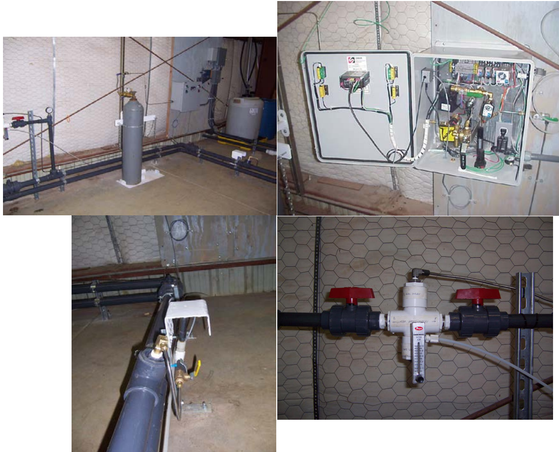
Figure 2-2. Carbon Dioxide Gas Flow Control System for pH Adjustment (Clockwise from Top Left: Liquid CO 2 Supply Assembly; Automatic pH Control Panel; CO 2 Membrane Module; Port for pH Probe)
