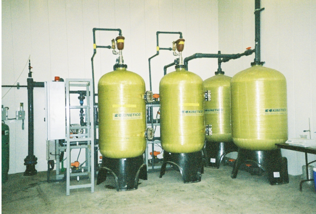
Figure 3-1C. 140-gpm Macrolite® Pressure Filtration System by Kinetico (Clockwise from Left: Control Panel, Macrolite® Filters, and Contact Tanks)
