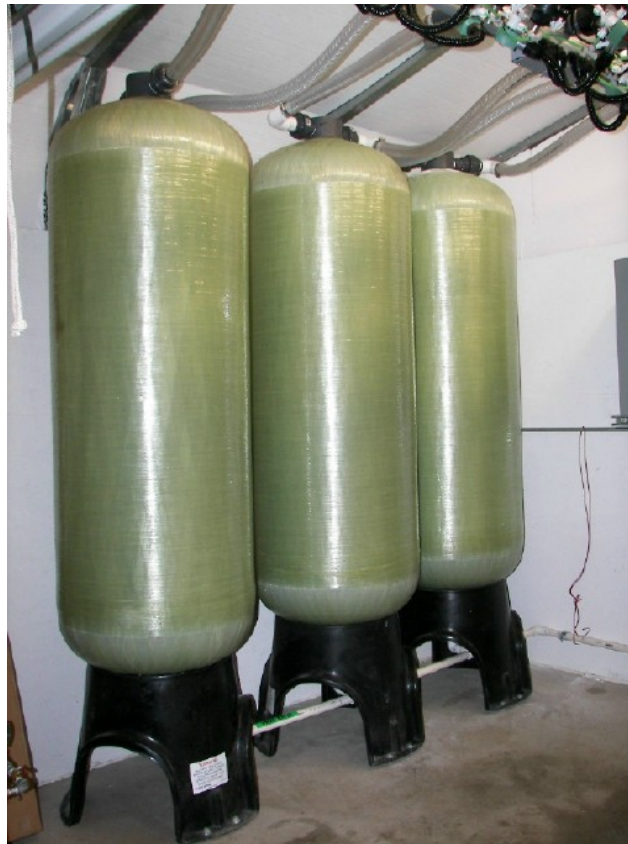
Figure 3-1B. 35-gpm Birm®/Filox™ and Adsorbsia™ GTO™ System by Filter Tech
