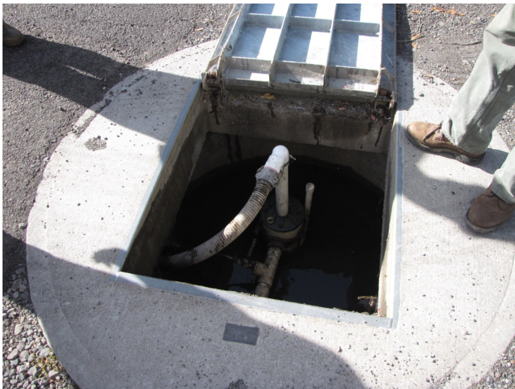
Photo 5. In-well stripping well IWS-6.
