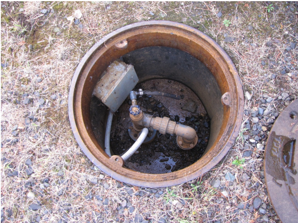
Photo 4. Extraction well PB-1B.
