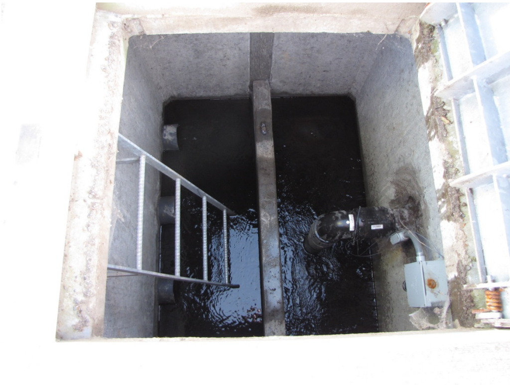
Photo 7. Infiltration gallery vault.
