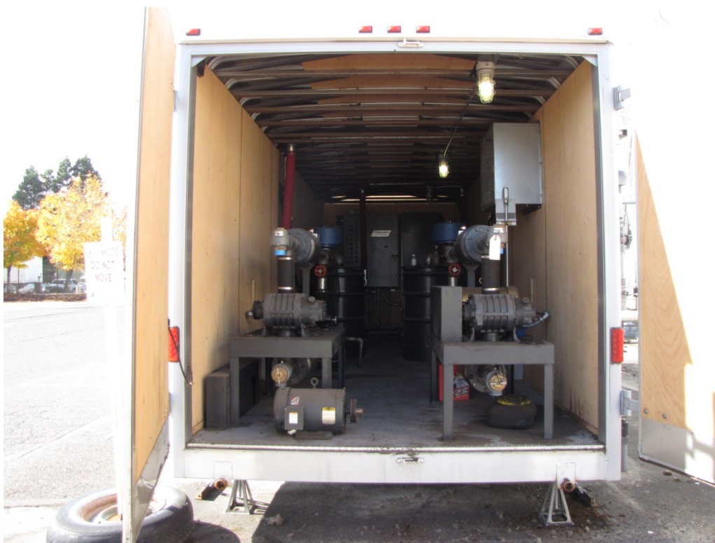
Photo 6. Blowers for IWS and SVE system.
