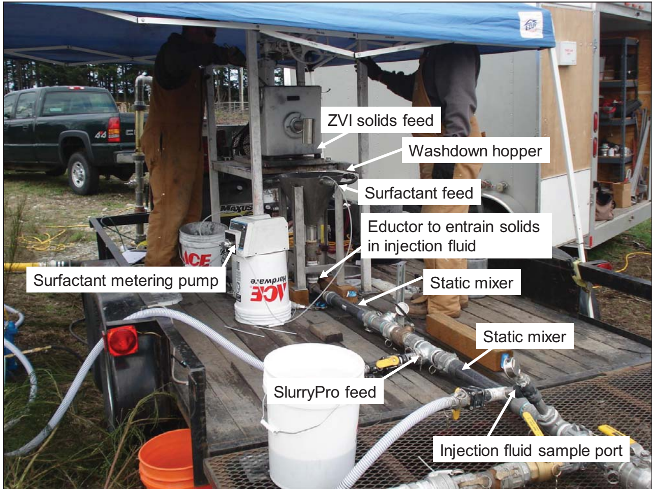
Figure 5-12. ZVI Injection System.
