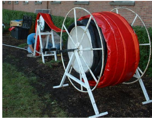
Figure 2-4: FLUTE™ Installation at the WVA
