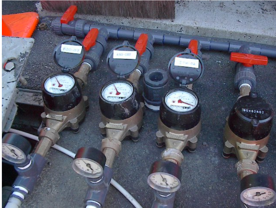
Figure 3.14 Injection system manifold showing separate control valve and flow totalizer for each injection well.
