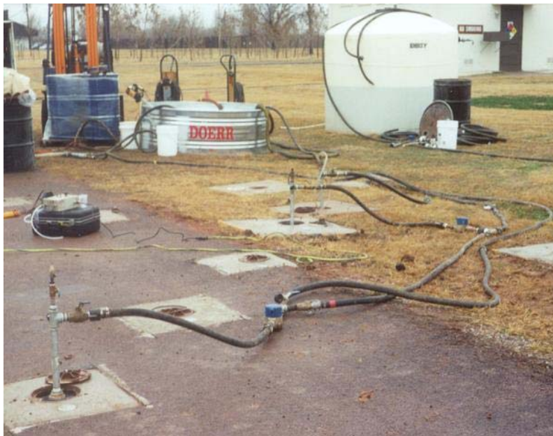
Figure 3.11 Typical injection system layout showing injection wells, feed lines with flowmeters and control valves, injection pump, emulsion mixing tank, and makeup water tank.
