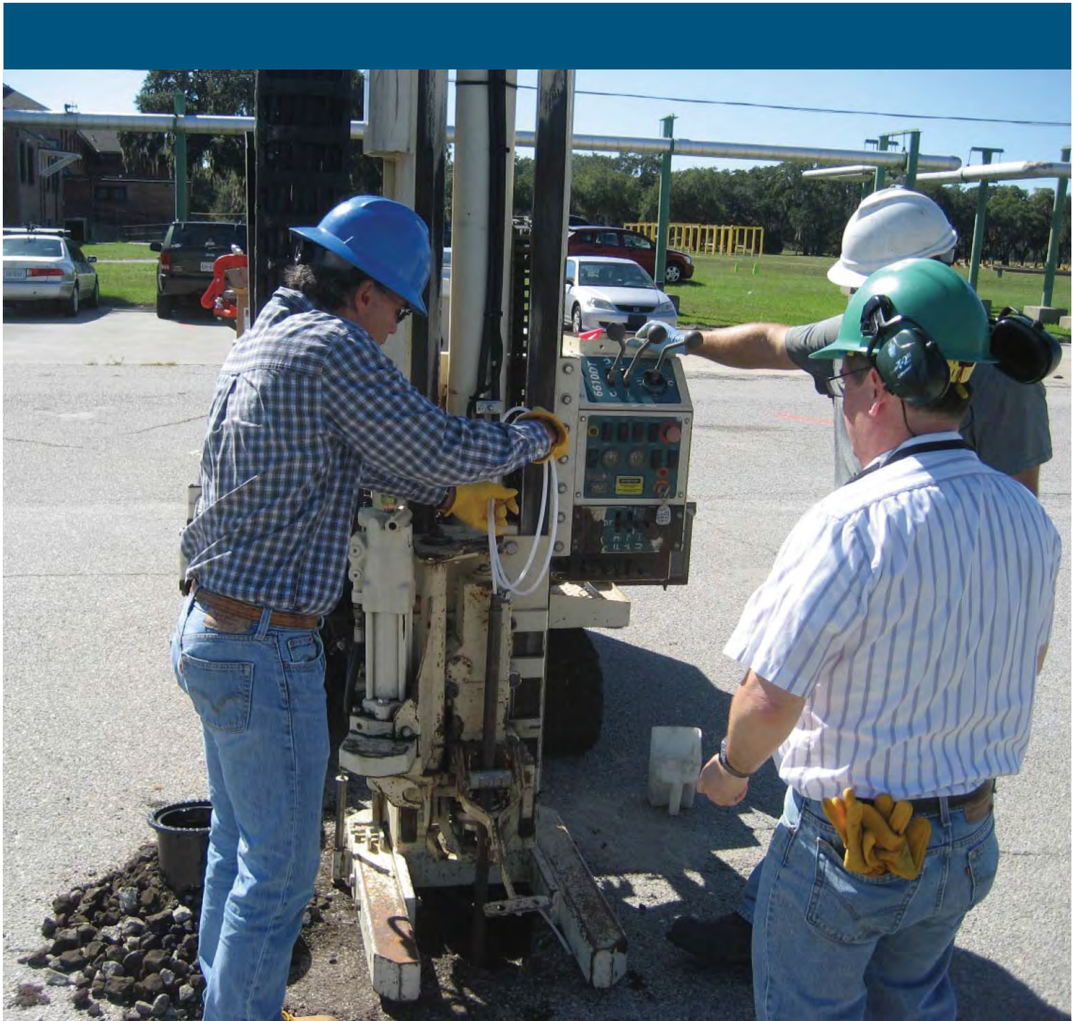
Photo 11. Installing the micro-well well screen and tubing by threading it through the Geoprobe rod to the target depth.
