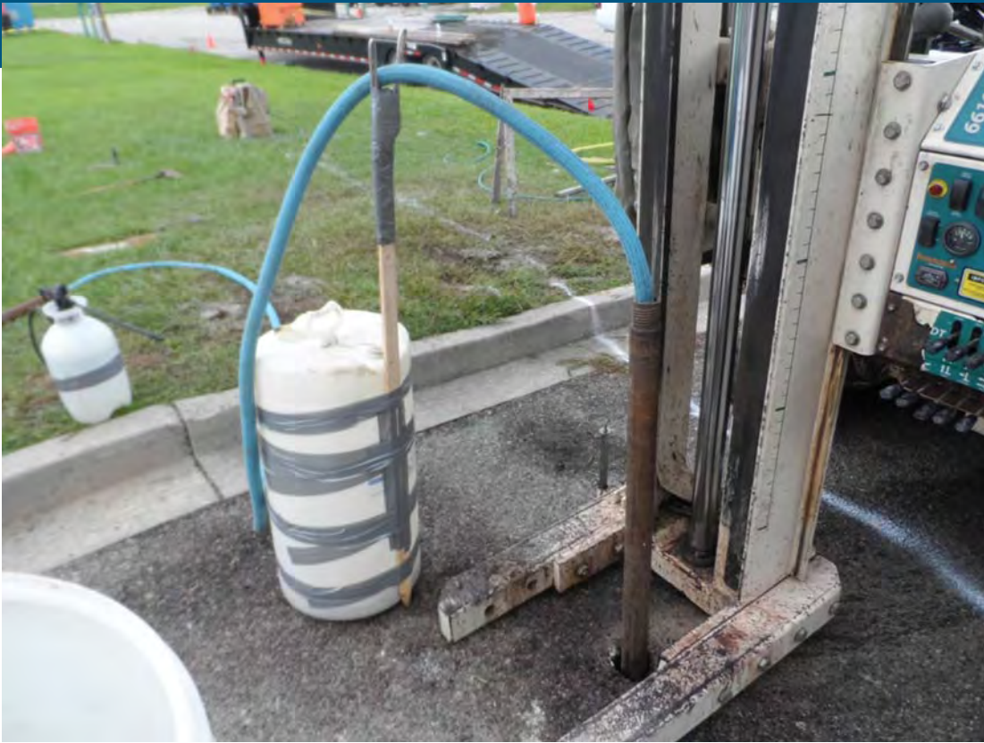
Photo 26. Oxidant injection at one location in the drive-through to the dry cleaner.
