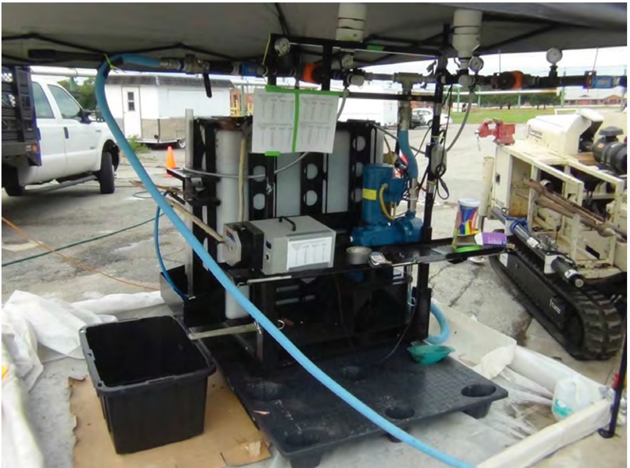
Photo 21. The oxidant injection system under a rain/shade canopy with 2 injection arms and secondary containment.
