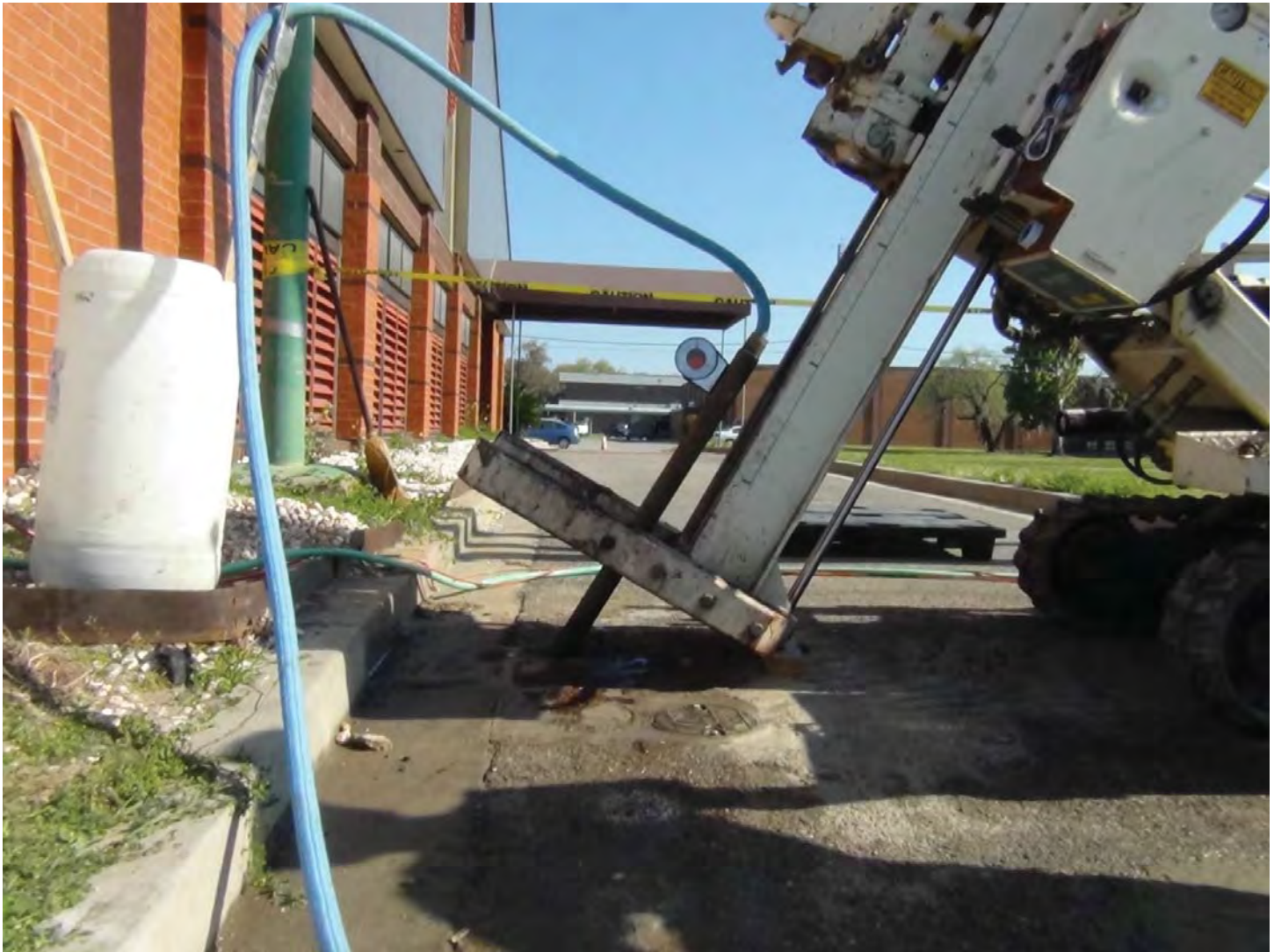
Photo 29. Direct-push at an angle of the injection tip to access the subsurface corner of building 192 in the drive-through of the dry cleaner. This technique was used to avoid the “mat apron” concrete foundation extending 5 ft from the building.
