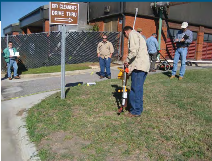
Photo 5. Utility notification prior to subsurface activity at Site 45 involved detection of utilities and marking. Marked utilities included a high pressure 8 inch water main (blue), communication line (orange), high voltage (230V) power line (red), storm and sanitary sewers (green). The approximate mid-line of the CVOCs plume was marked by the research staff (yellow).
