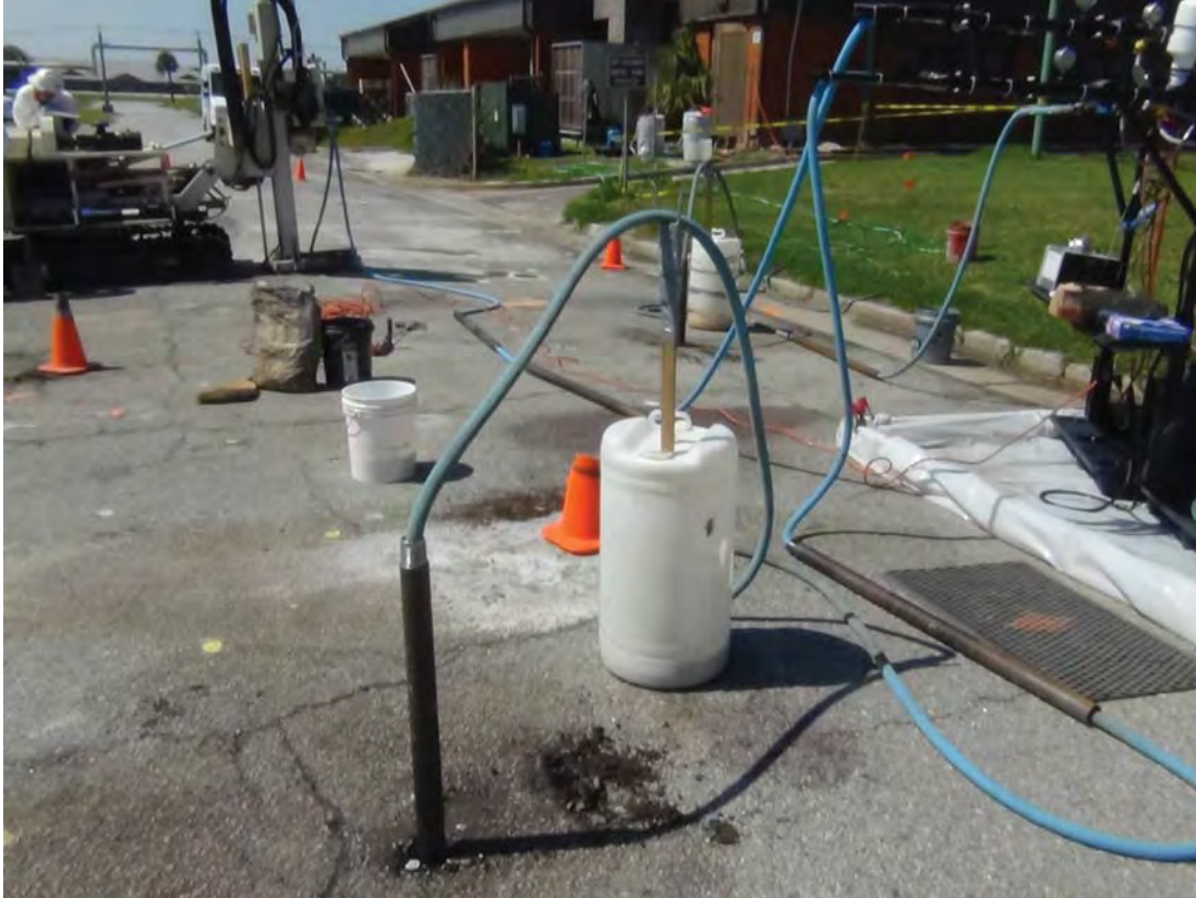
Photo 27. Simultaneous injection of oxidant into three locations on Kyushu Street while avoiding subsurface utilities. Facing the west, these injection locations straddle the communication line and flank the south side of the 8" high pressure water main and 230V high voltage line.
