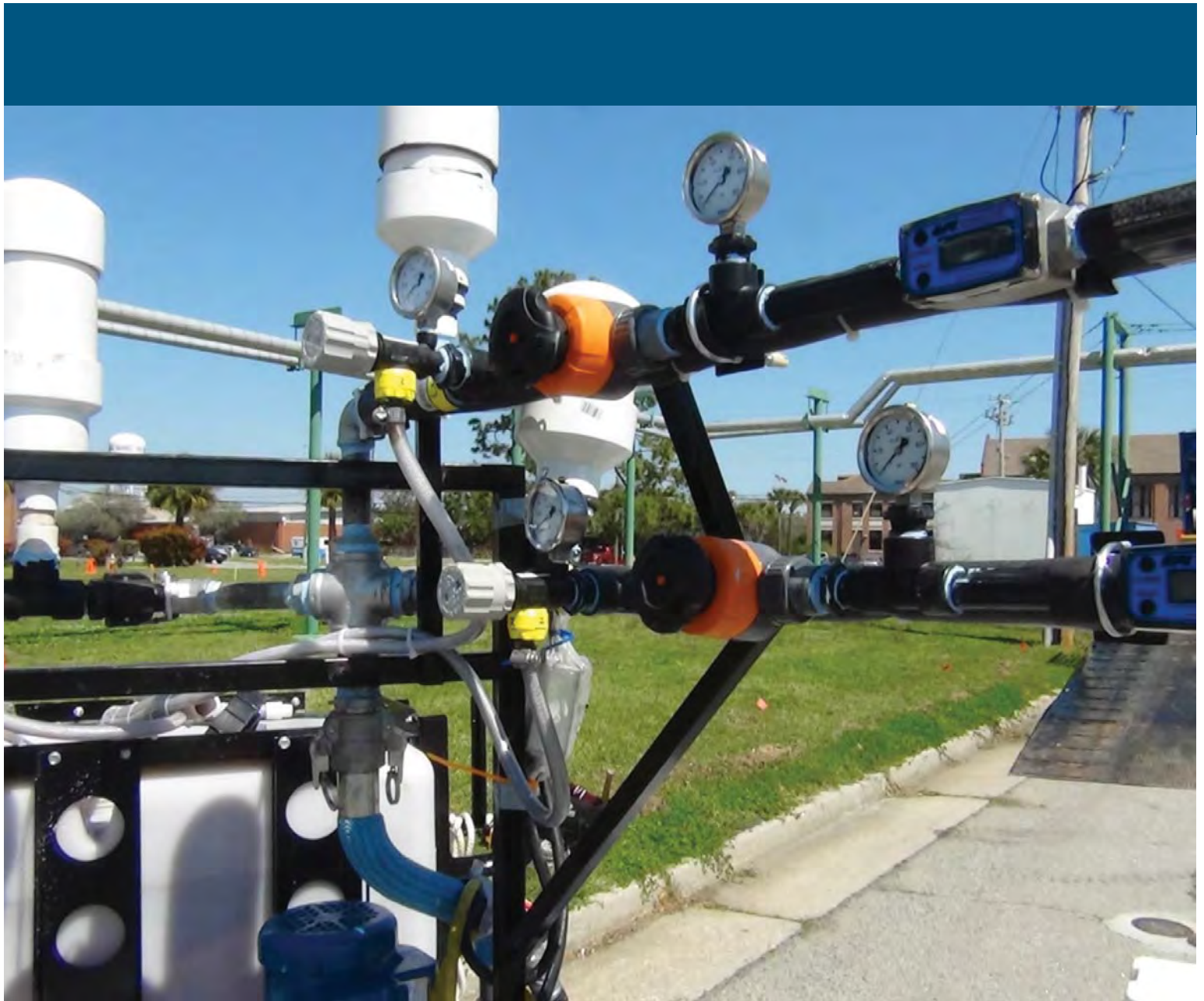
Photo 22. Three (3) oxidant injection arms in use at site 45. Each is equipped with flow dampener, pressure gauge, pressure relief valve and return line, flow control valve, pressure gauge, in-line flow totalizer, and on the end is the (not shown) emergency shut-off valve.
