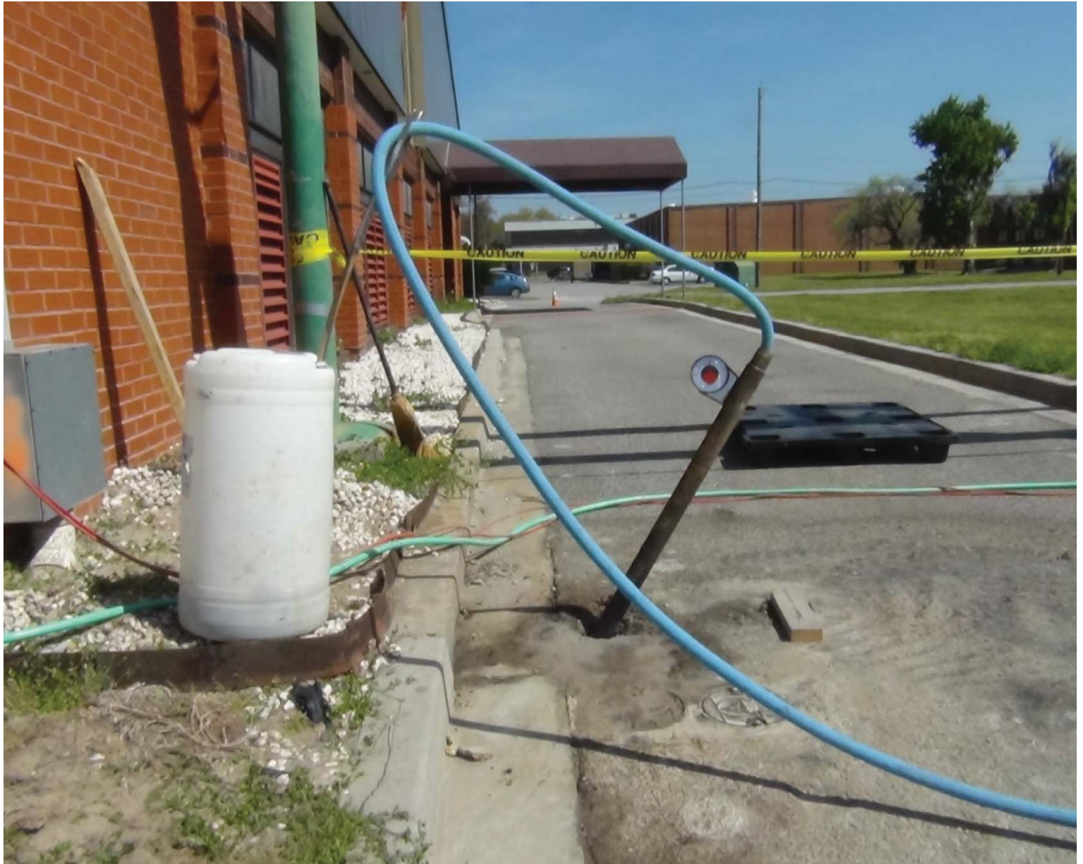
Photo 30. Direct-push of oxidant under corner of the Bldg. 192 into the source area associated with the former leaking sanitary sewer line in this area. This was performed while avoiding the communication lines (orange-marked utility box is the communication line), and the overhead steam line supported by the green post in the background of the photo.
