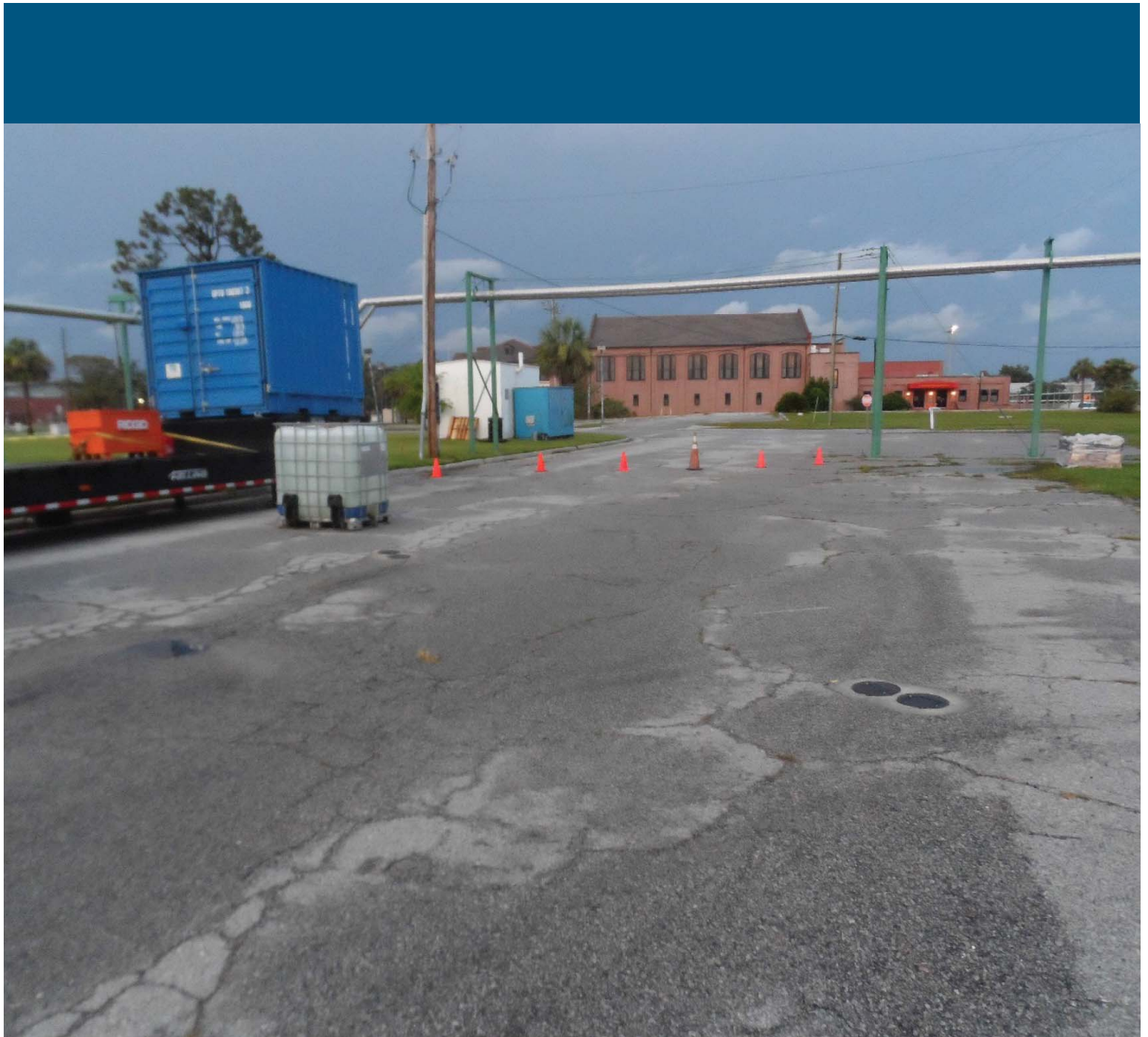
Photo 25. Access restrictions along Kyushu Street while oxidant handling and injection activities were ongoing.
