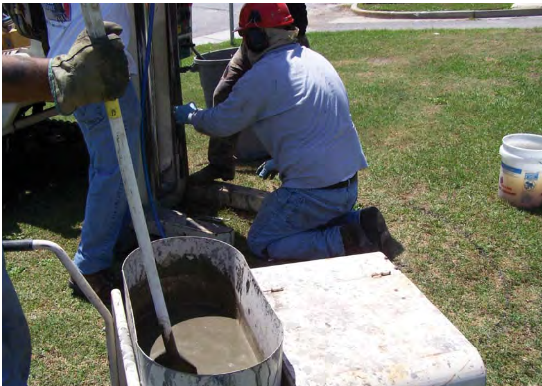
Photo 8. Preparation of cement-bentonite grout using GeoProbe grout pump. The grout was pumped into the bottom of boreholes where soil cores were collected. A tremie tube and a “bottom-up” method was used to properly seal abandoned soil coring locations.
