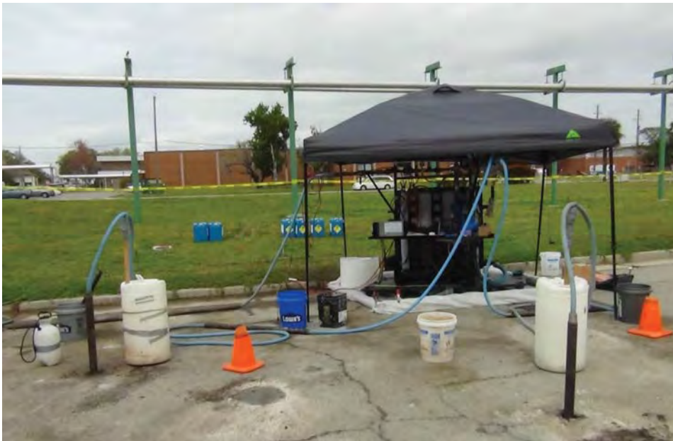
Photo 28. Rain/shade canopy used for injection pallet while oxidant is delivered to three locations.
