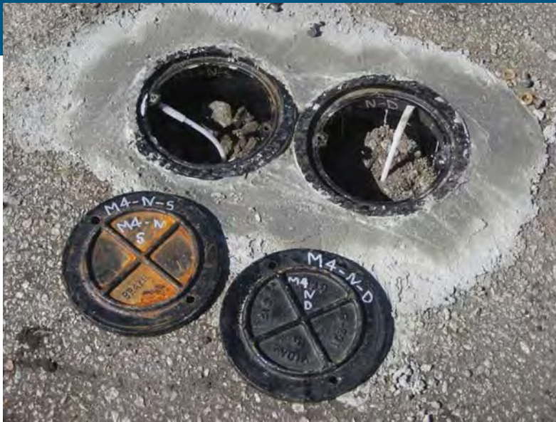
Photo 14. Construction of flush-mounted paired micro-wells ( i.e. , shallow and deep). Paired micro-wells with identification markings M4-N-S and M4-N-D indicate monitoring transect 4, north side of the plume, shallow and deep intervals.
