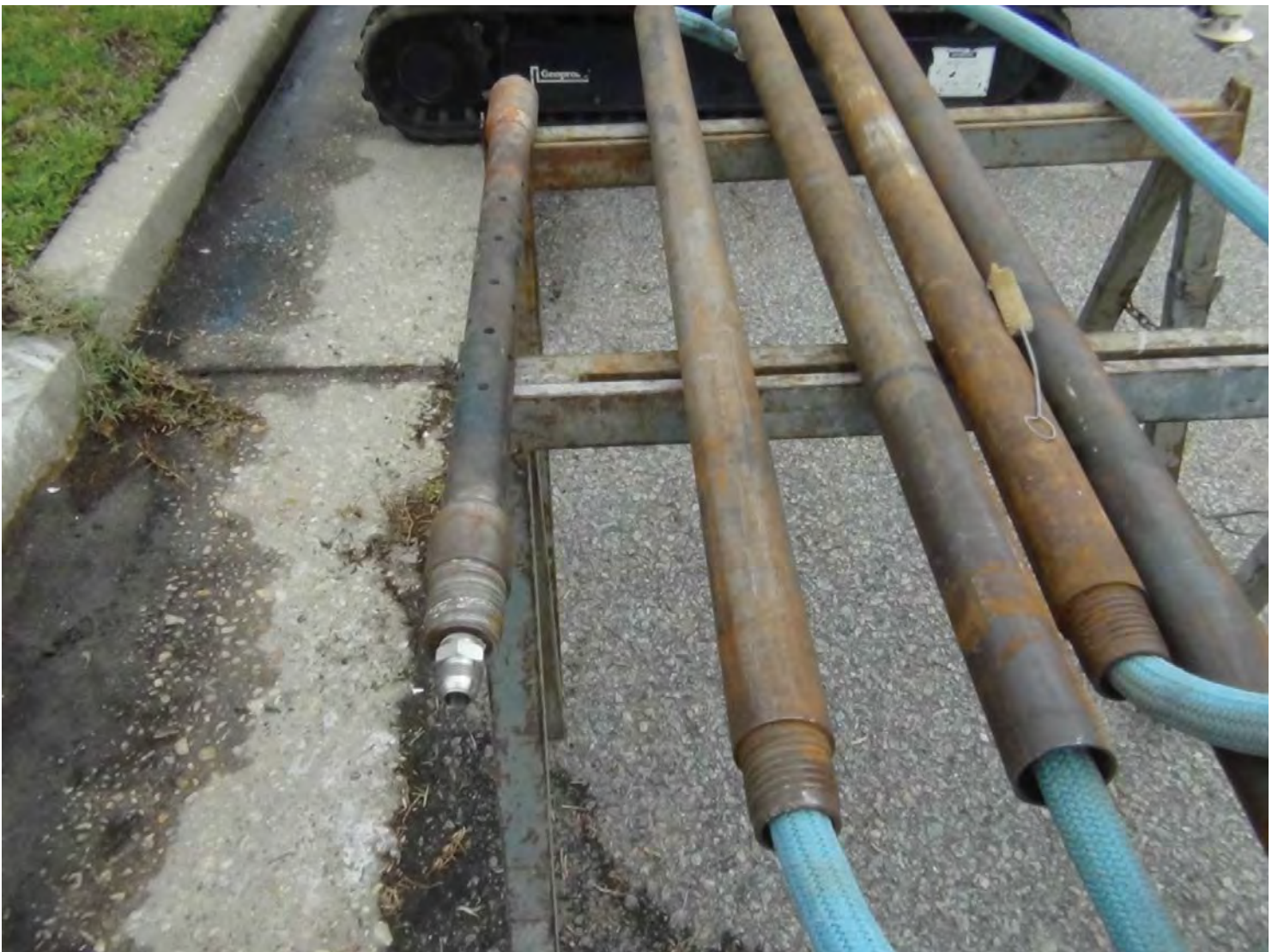
Photo 19. The injection tool with holes (left) for oxidant delivery into the subsurface is connected with corrosion-resistant stainless steel fittings. The corrosion-resistant, oxidant delivery line (blue) is Pureflex Ultraflex PTFE (45-60 ft in length) and is a convoluted hose with polypro braid.
