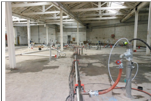
FIGURE 6: Above Ground Pipework.
