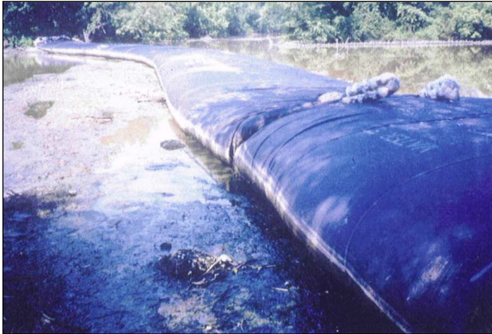
a. Geotextile Water-Filled Tubes Being Used as a Temporary Dam to Contain Dredged Material until it had Sufficiently Dewatered so that Marsh Planting Could Take Place at Kenilworth Marsh on the Anacostia River, Washington, DC, in 1993; the Tubes were Removed once the Material had Consolidated, and the Site was Planted
