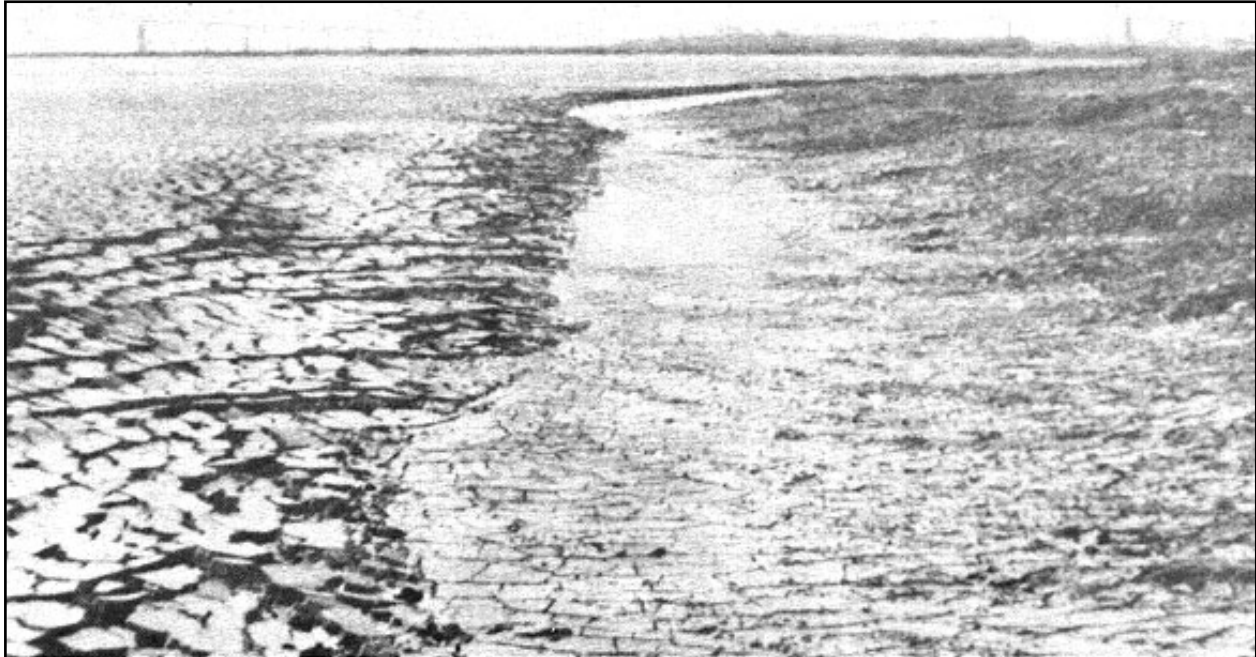
Figure 4-31. Shallow Initial Perimeter Trench Constructed by a Dragline Operating from the Perimeter Dike
