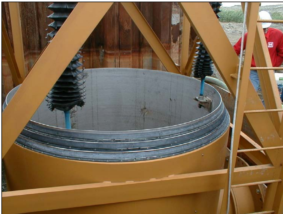
b. Closeup of Adjustable Weir
