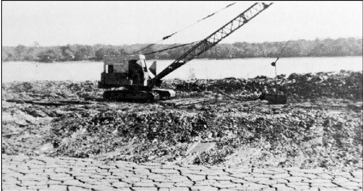
Figure 4-32. A Small Dragline on Mats, Working on a Berm, Deepens a Shallow Perimeter Trench
