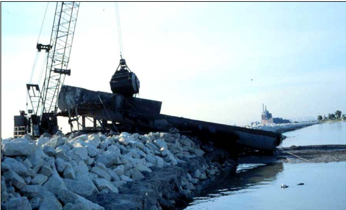
Figure 4-11. Placement Using a Chute Fabricated from Railcar Tanks for Direct Mechanical Placement into a CDF
