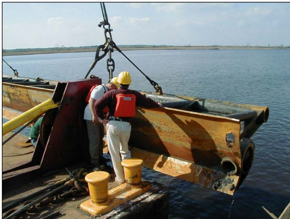
Figure 2-41. Bed-Leveler Suspended by an A-Frame on a Work Barge (Photo Courtesy of Great Lakes Dredge and Dock Company)
