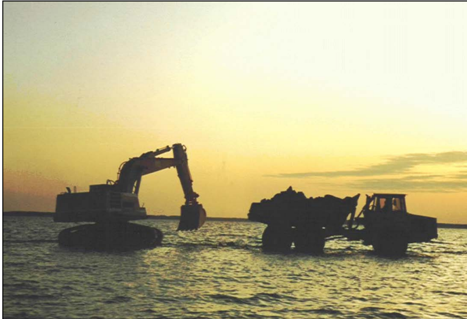
a. Construction of the Riprap and Dredged Material Detached Breakwaters to Break Wind Fetch and Wave Energy, Approximately 125 m (400 ft) Offshore in Shallow Water at Eastern Neck National Wildlife Refuge
