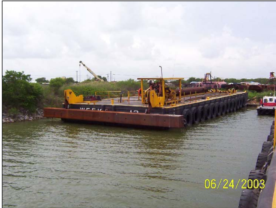
Figure 2-40. Bed-Leveler Suspended from a Work Barge (Photo Courtesy of Weeks Marine, Inc., Cranford, NJ)
