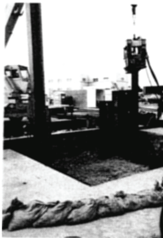
Figure 5. Sheet piles emplaced using a vibrating hammer (after USACE (1997), courtesy of PRC Environmental Management, Inc. (1996))
