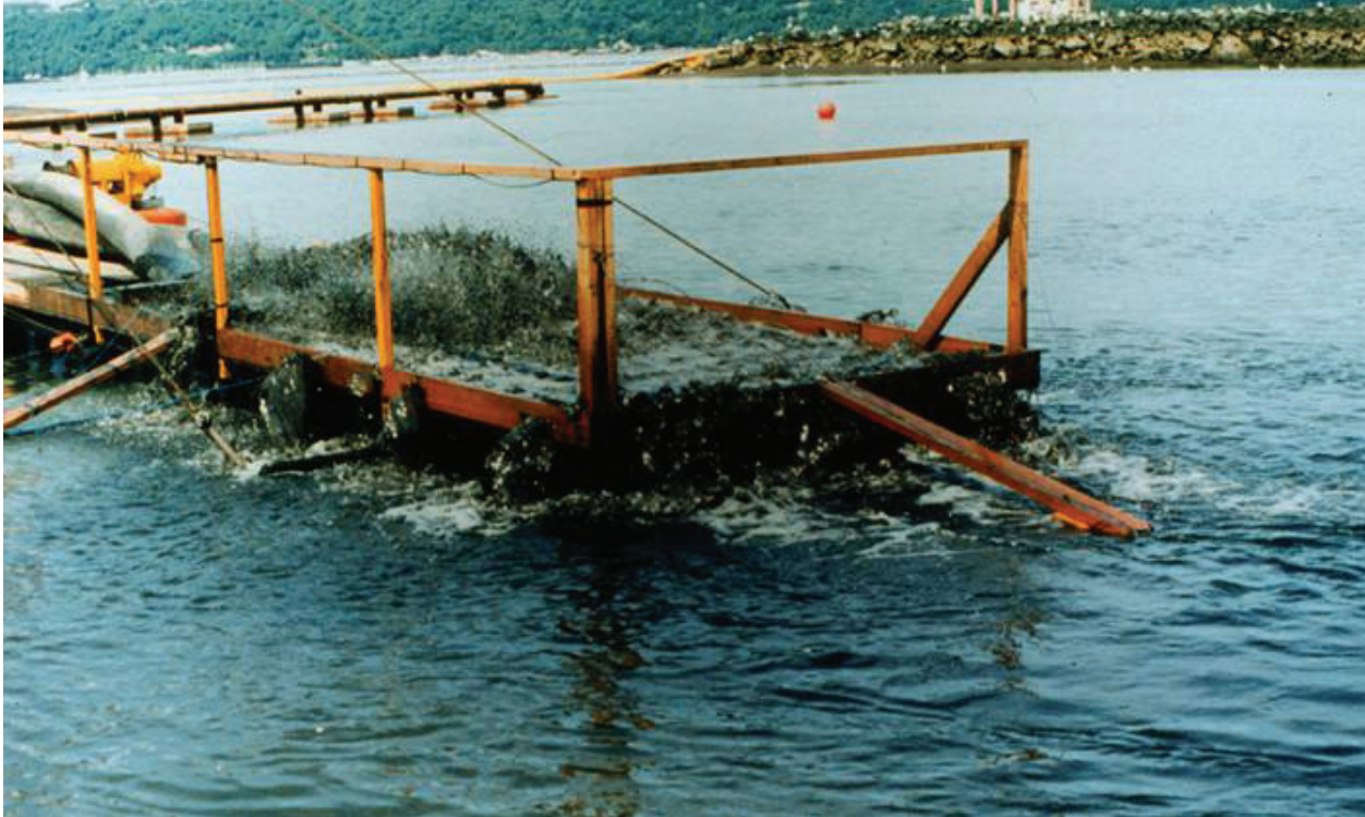
Figure 9. Spreader box or sand box for hydraulic pipeline discharge, Simpson Kraft Tacoma, Puget Sound
