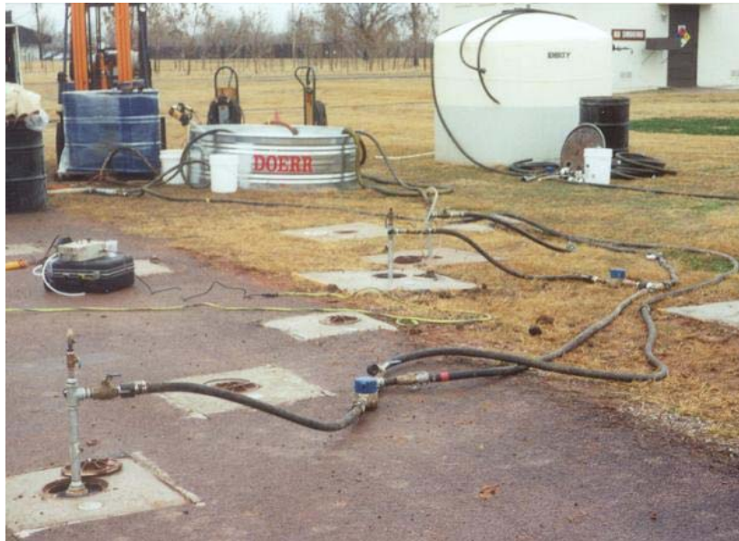
Figure 5.6 Typical Injection System Using a Field Prepared Emulsion, Altus AFB, Oklahoma
