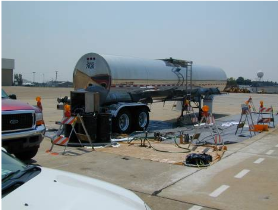
Figure 5.3 Typical Injection System Layout for Pure Edible Oil, Naval Support Activity Mid-South, Tennessee
