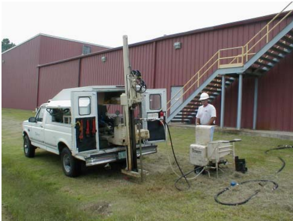
Figure 1.7 Direct Injection of Pure Edible Oil through Geoprobe® Rods Using a Grout Pump
