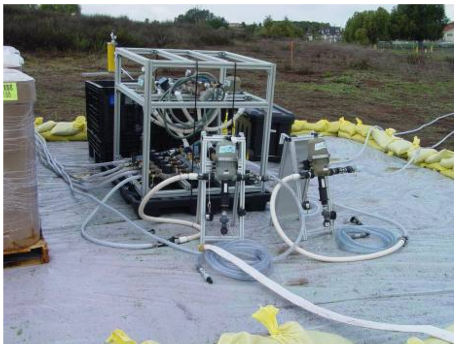
Figure 5.11 Proportional Feed System for a 10-Line Injection System (Photo courtesy of Remediation and Natural Attenuation Services, Inc.)
