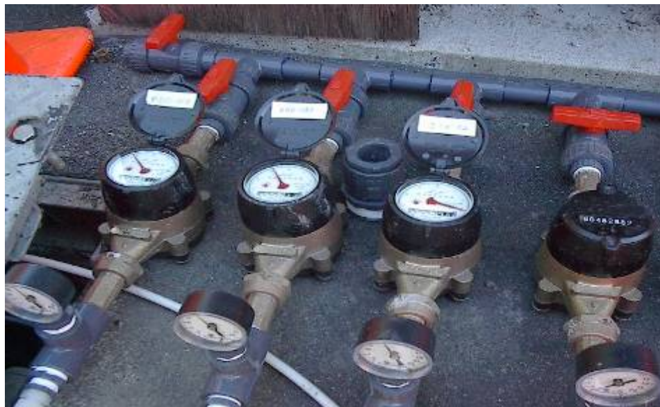
Figure 5.10 Injection System Manifold Showing Separate Control Valve and Flow Totalizer for Each Injection Well (Photo courtesy of EOS Remediation, Inc.)
