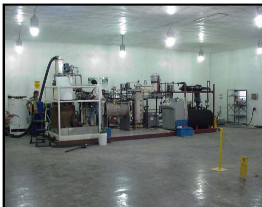
Typical SET™ Plant
