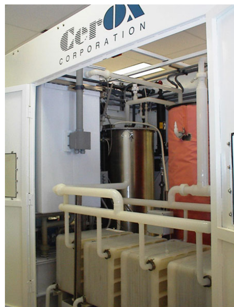
CerOx™ treatment system, Source: Ref. 15
