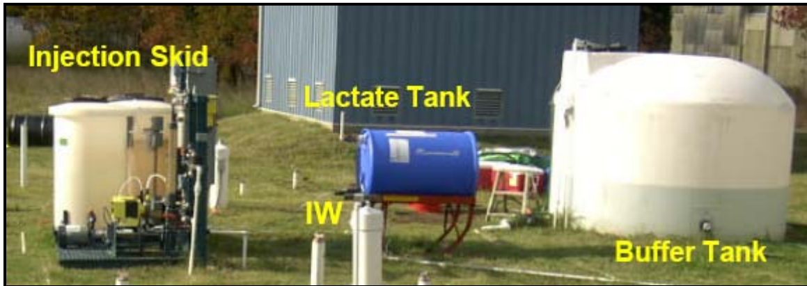
Figure 12. Photograph of the Above Ground Infrastructure: The Injection Skid, Lactate Tank and Buffer Tank. (Reprinted from Hatzinger, 2004)
