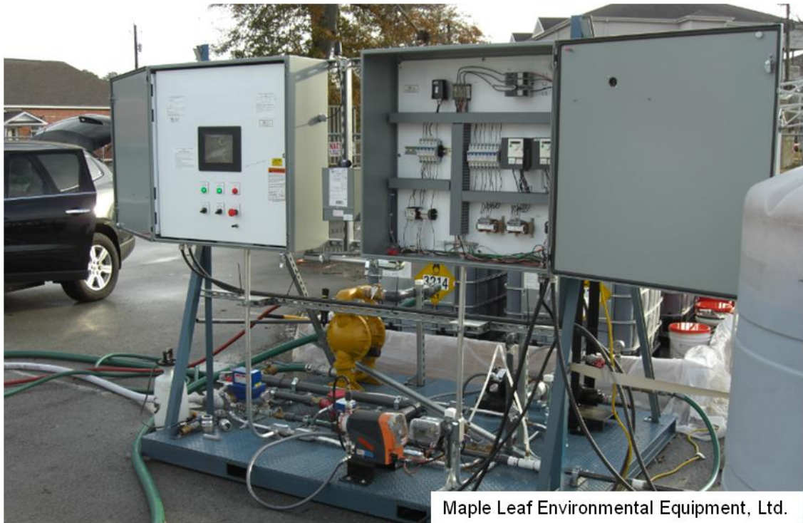
Figure 5-14. Automated process control system.
