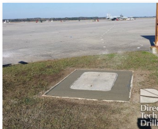
Horizontal air-spargewellhead at Eglin AFB (EDTD 2023)
