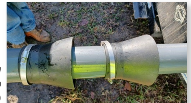
Formation packer/shale trap (Geosyntec 2021)
