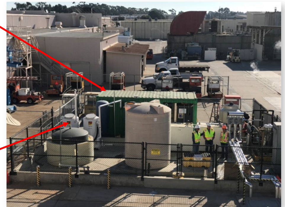
Remediation system compound (NOREAS 2018)
