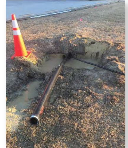
Horizontal well head with grout tremie pipe (FPM Remediations 2018)
