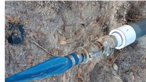
HW head flushing connection (Geosyntec 2021)
