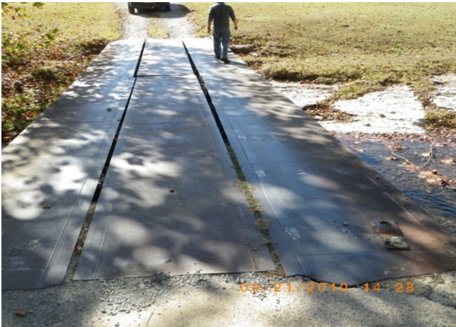
Mercury Cell Plate Bridge
