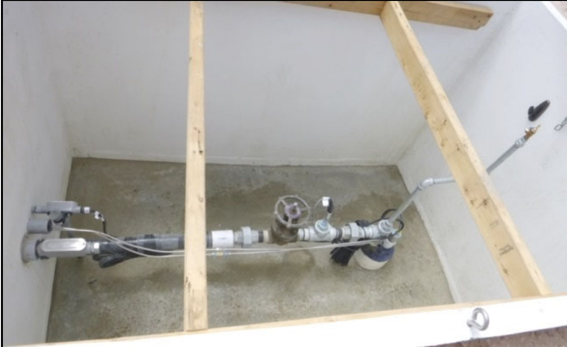
Description: Completed extraction/injection well vault and wellhead manifold.
