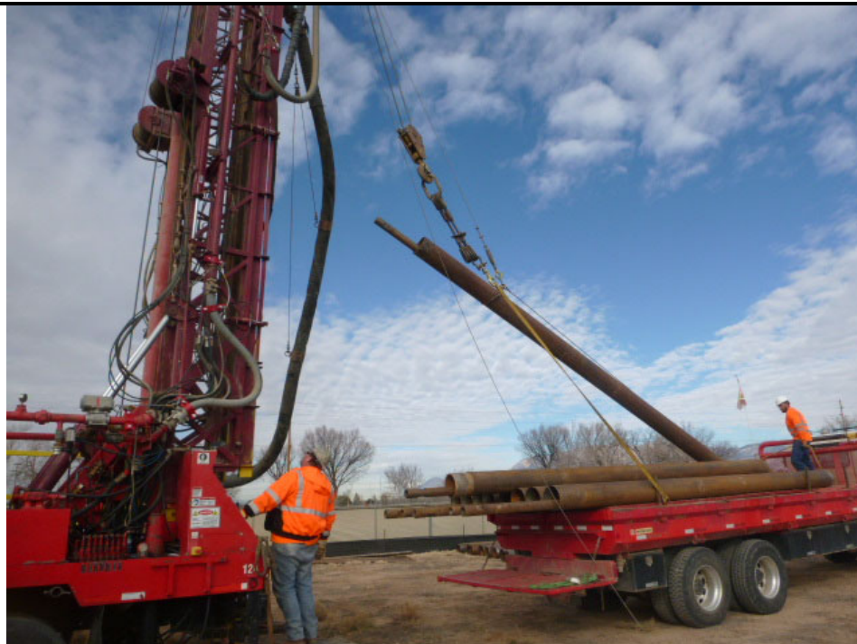
Description: Cascade drilling with ARCH rig; lifting drive casing and drill string.
