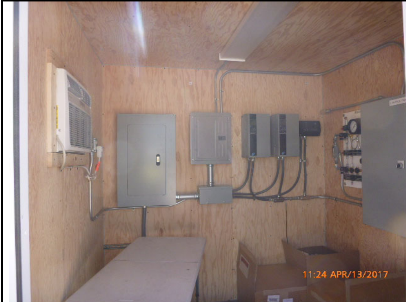
Description: Interior of recirculation system control room.
