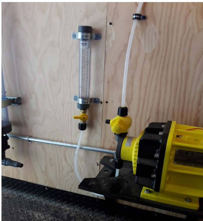
Description: Chemical feed pump (right) and calibration column.
