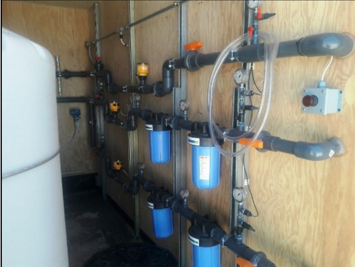
Description: Interior of conex box recirculation system (wet side); showing extraction and injection well piping, amendment tank, flow meters (yellow), pressure transmitters, emergency stop button, and blue filter canisters.
