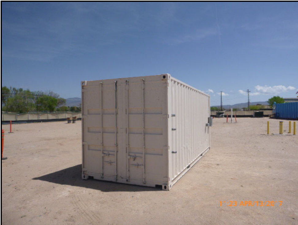
Description: Recirculation system conex box prior to connection to electrical and conveyance piping.
