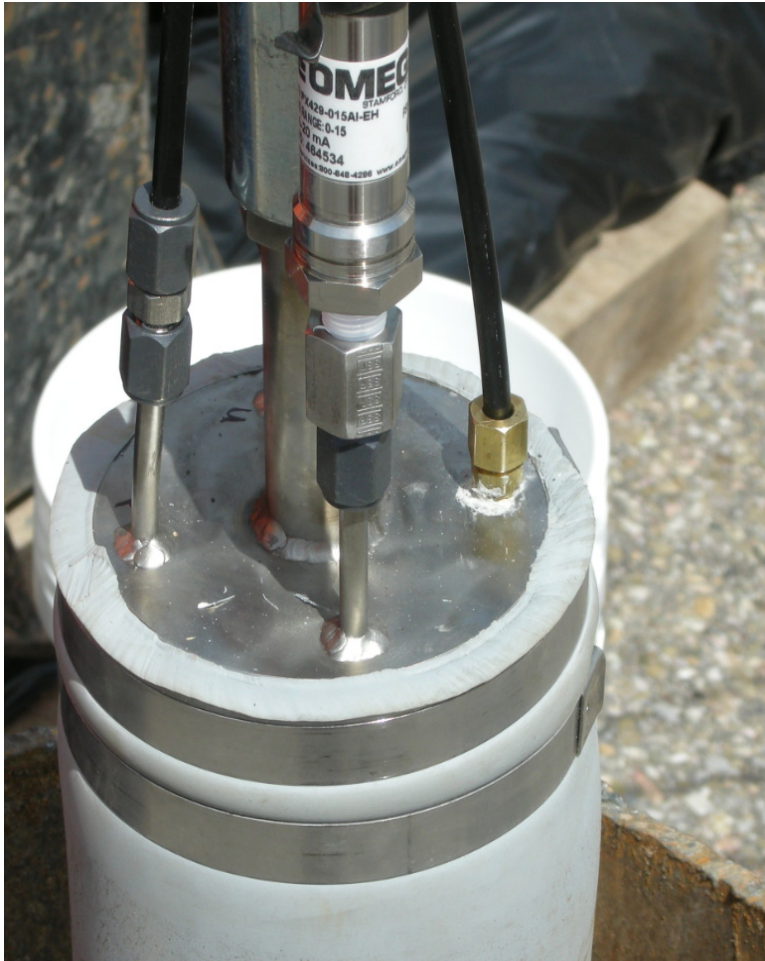
Figure 2.2-4 Top of the permanent packer showing the OMEGA pressure transducer, one sample line, and the nitrogen inflation line
